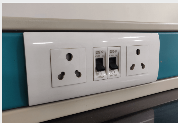
6/16 Amp Sockets with MCB
